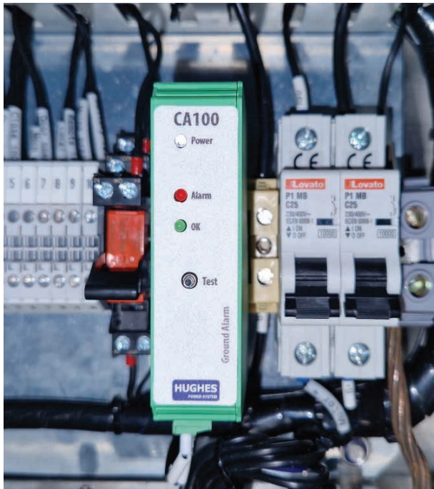
Installation in the motor drive cabinet
